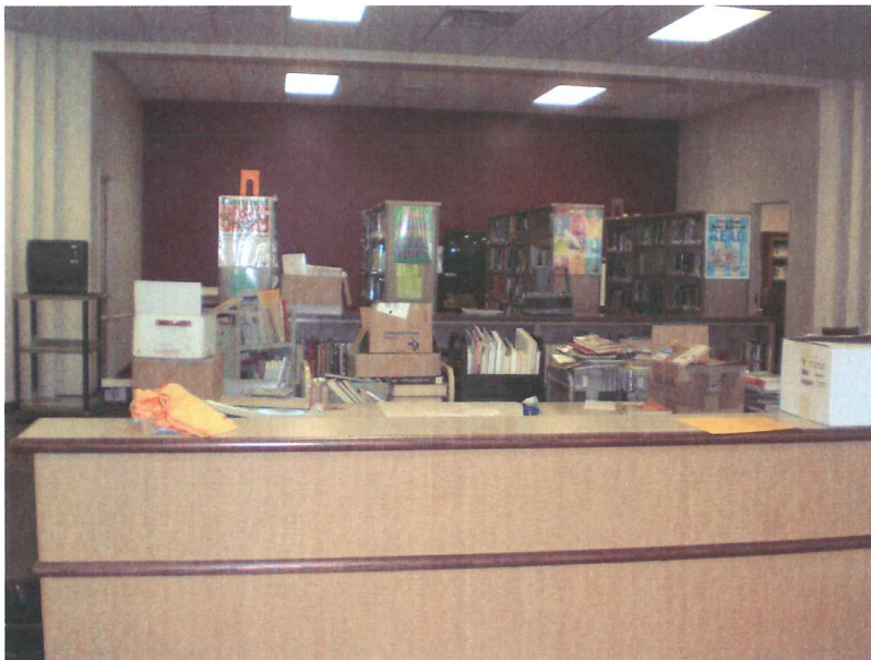
The Library was completely gutted. Two storage rooms flank the large desk area.
